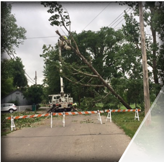
Becker County storm damage in July 2017.
