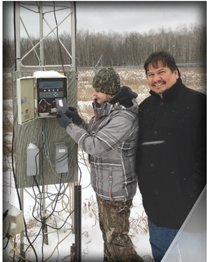
Duane Oothoudt, Leech Lake Band of Ojibwe's Emergency Management Director, and Carma Huseby, Division of Resource Management, check on the cellular transmitter now installed on an existing weather tower.
