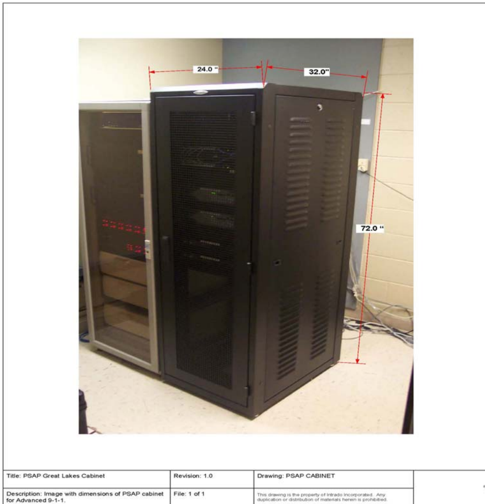
Figure 1: PSAP Equipment Cabinet
