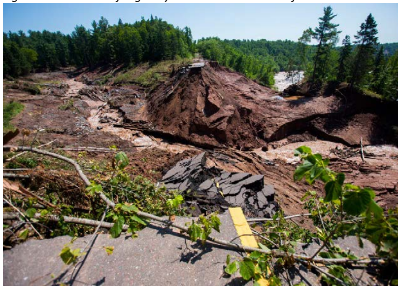
Figure 42. A section of Highway 210 was washed out after a dike was overtopped at Forebay Lake
