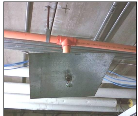
Exhibit 1: “Heat collector” improperly utilized in lieu of proper sprinkler placement.
