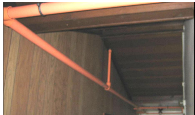
Sloped (not horizontal) ceiling. Pipe centerline exceeds the 7½-in maximum.
