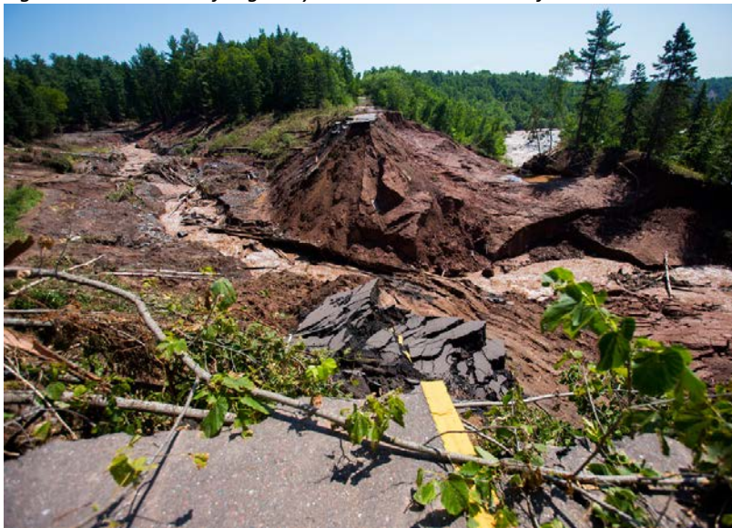
Figure 42. A section of Highway 210 was washed out after a dike was overtopped at Forebay Lake
